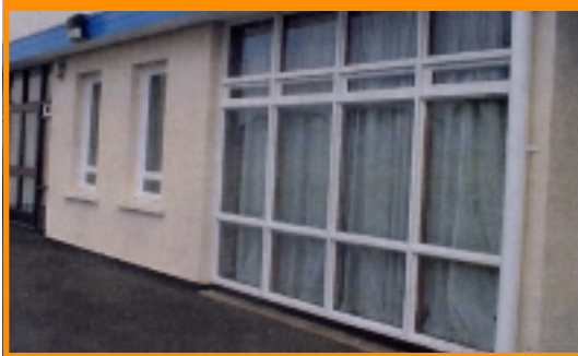
Low Level Glazing on walls
