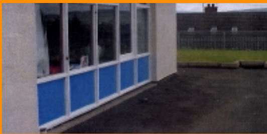
Windows facing onto playground - Deemed High Risk due to the type of activity carried out close to glazed area
